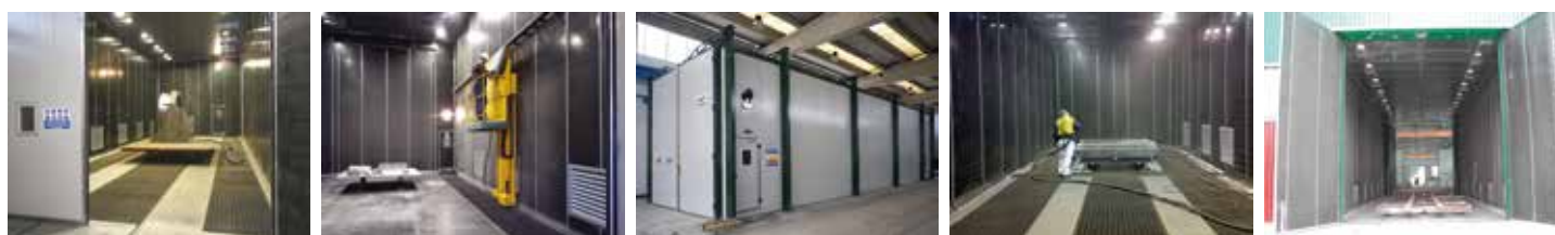
With scraper and e cochlea inside the building
